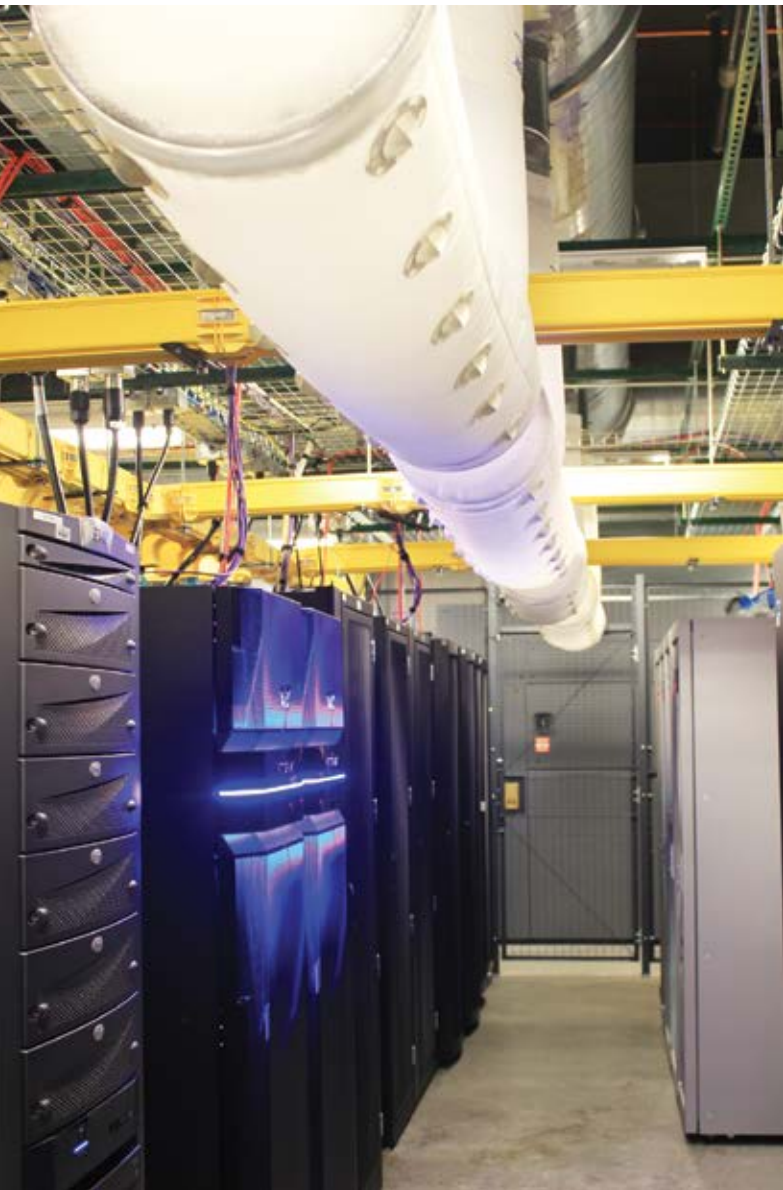
⌘ Data centers pose numerous ventilation challenges.
